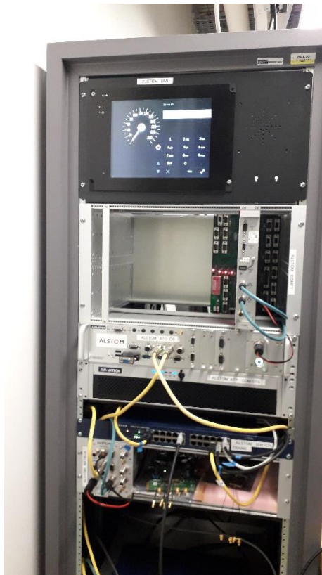
Figure 64: Train part of Alstom cabinet
