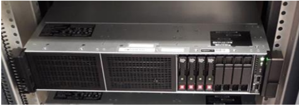
Figure 18: HP Gen-10 equipment installed in WP4 lab for IMS/MCx functions hosting
