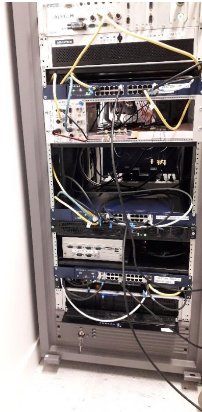
Figure 65: Ground part of Alstom cabinet
