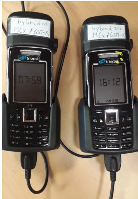
Figure 24: GSM-R handsets installed in WP4 lab
